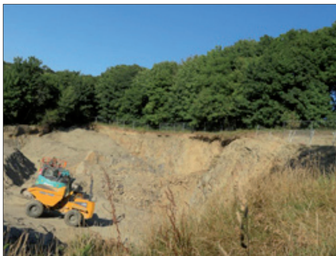
One of the landslips at Lock's Hill
