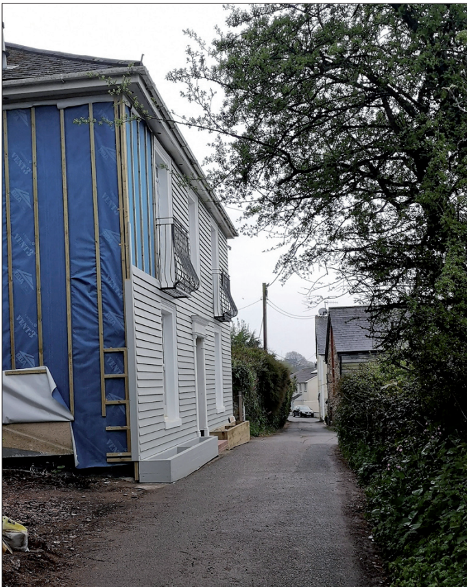
Retaining Dennings House will make the road too narrow to cope
