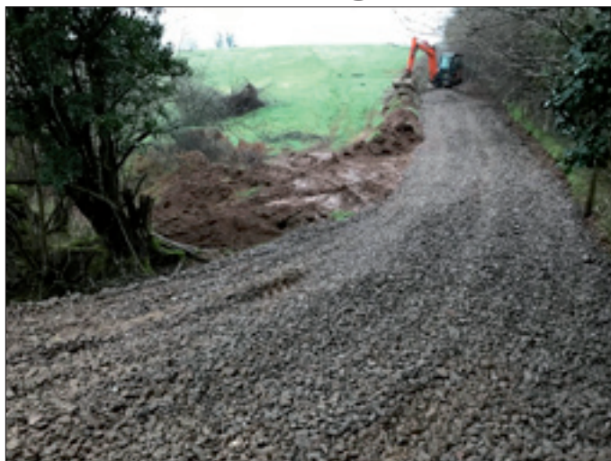
The track, cut in damagingly close to the hedgerow
