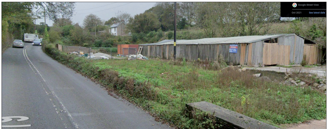
Wood framed Milk Parlour, repaired and closed with new boarding to gain Class Q permitted development rights.
